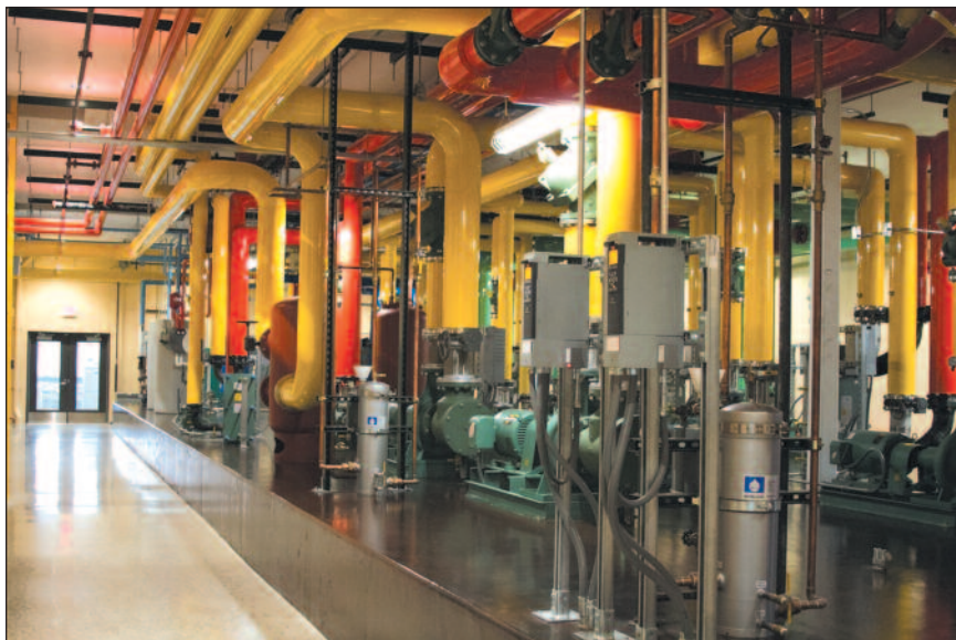
Color-coded pipe insulation allows visitors to follow system flow and operation. Each color has different meanings, specific to the loop it's part of. Red is specific to the heating loop, while dark blue identifies chilled water. ITEC's mechanical system includes six different colors.
