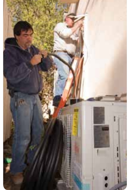
Matt Madrid flares the refrigeration lines to install on the condenser (front), while Miguel routes the refrigeration lines through two-inch hole at the home in downtown Santa Fe.
