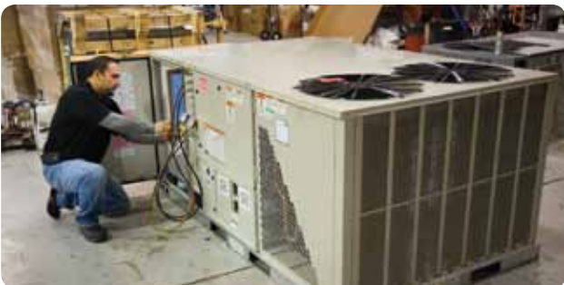
Service Technician/Lead Hospital Division Installer Eric Tafoya looks over a new McQuay package unit before installation at a local hospital facility.
