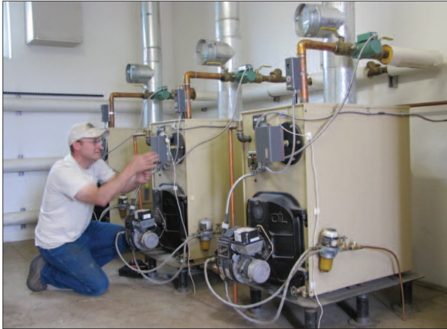
Joel Ballek wires in the Taco pump to the Aqua Stat at Eagle's Nest Condos in North Pole, Alaska.
