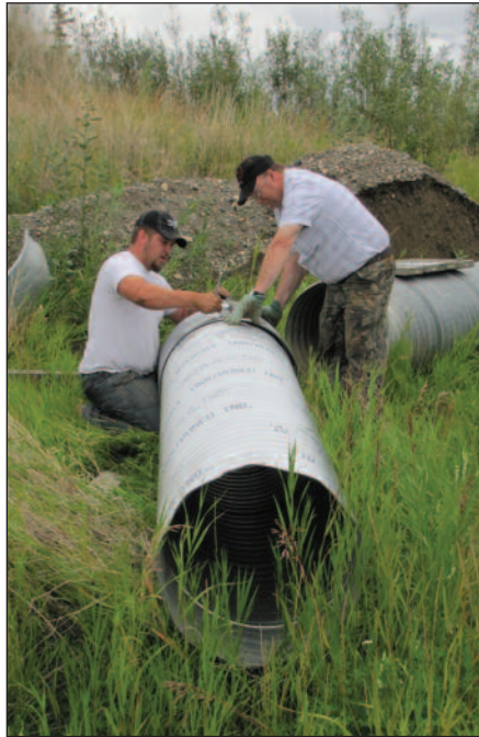
Jeff Ballek and his nephew Justin Ballek put together a culvert for a new subdivision off of Patriot Drive in North Pole.
