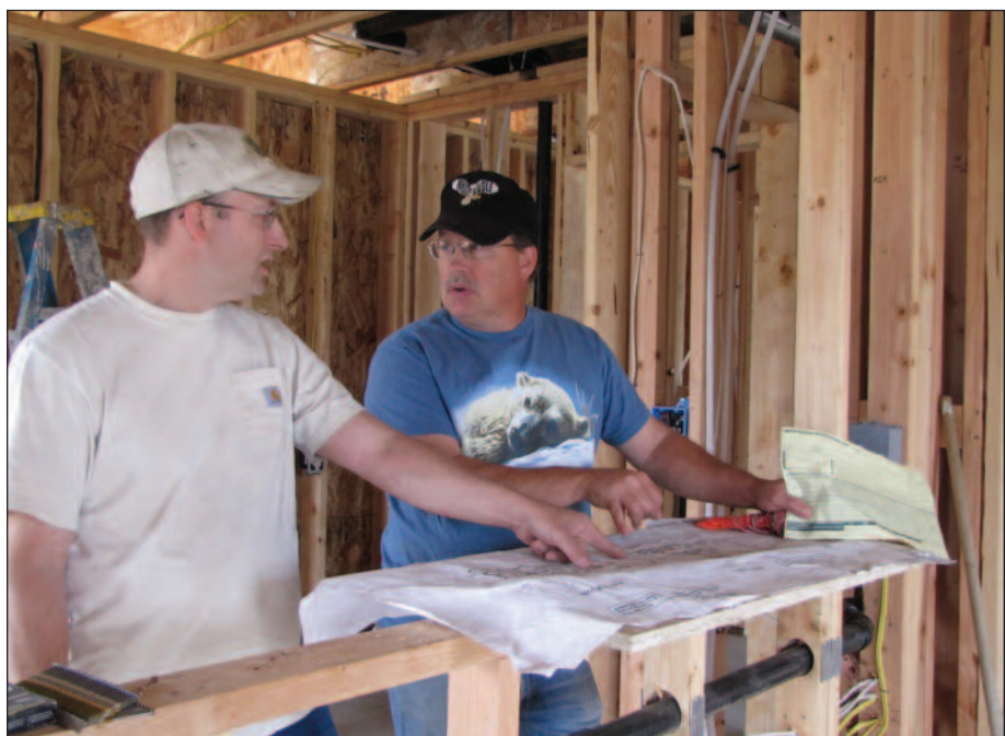
Joel and Jerry Ballek reading the blue prints for the domestic water and sprinkler system at Eagle's Nest Condos in North Pole.
