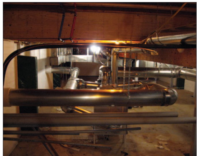
Round ductwork in the basement of the Center of Design Research provides both intake and exhaust for the ERVs, which are the backbone of the systems in the building.
