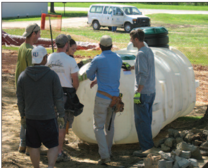
Hard working Studio 804 students gather around the 1,200-gallon rainwater catchment tank to take a break in the shade.
