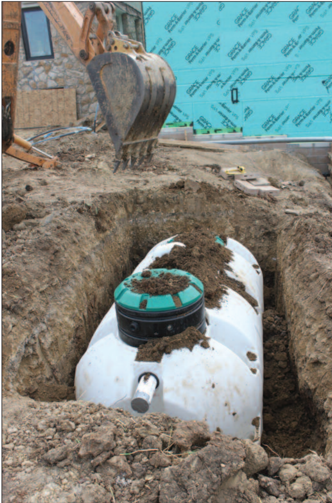
A 1,200-gallon tanks that serves as the storage for a Brae rainwater harvesting system is installed in the back yard of the Center of Design Research.
