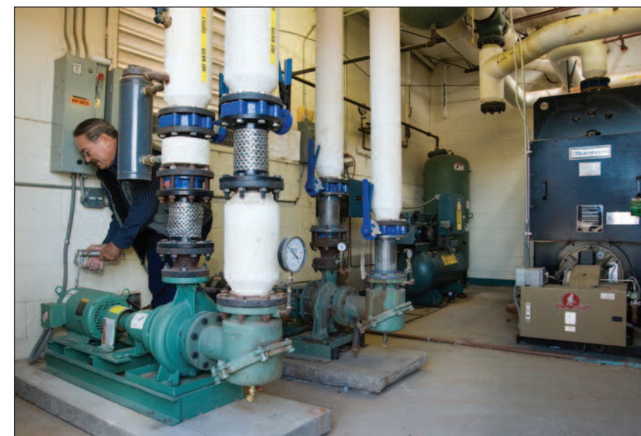
Joe greases Taco recirculating pumps at the K-4 campus of Pojoaque Valley Schools.
