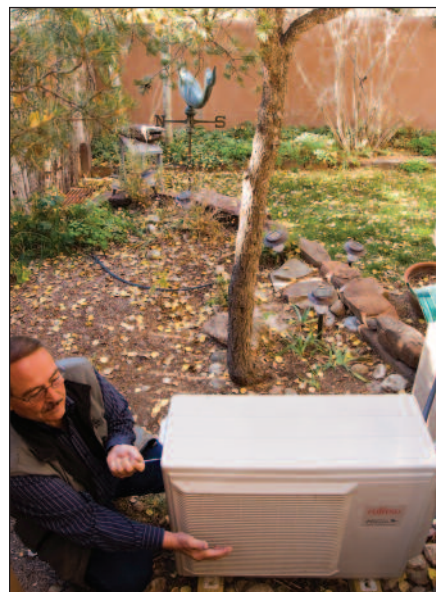
Joe Salazar performing routine maintenance inspection on one of the five one-ton Fujitsu heat pumps installed in a Santa Fe residence
