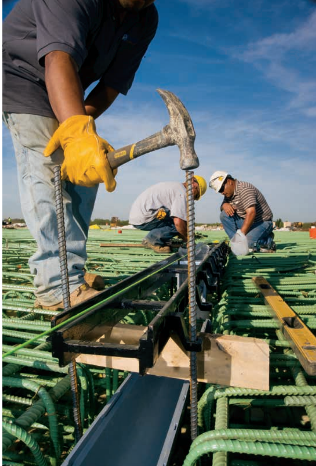
At a FedEx jobsite in Virginia, Dulles Plumbing Group installers set DeadLevel™ trench drain sections. Dave Hudgens, president of the commercial plumbing and mechanical contracting firm, knows firsthand how advanced drainage technology can save jobsite time, keeping a company ahead of schedule for a client that's literally racing the clock 24-7/365.
