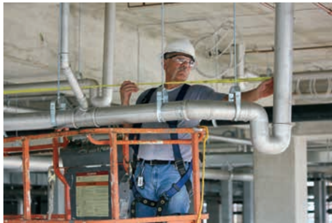
An installer with Gallo Mechanical connects Blücher stainless steel drainage sections at the Orleans Parish Prison in New Orleans.
