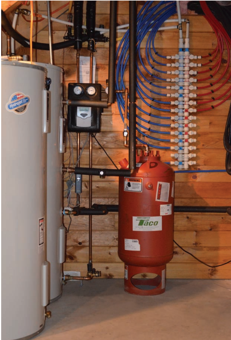
Even with advances in solar technology, some accessories will probably be on tap if a hydronic system is in the plans. Photo courtesy of Taco.
