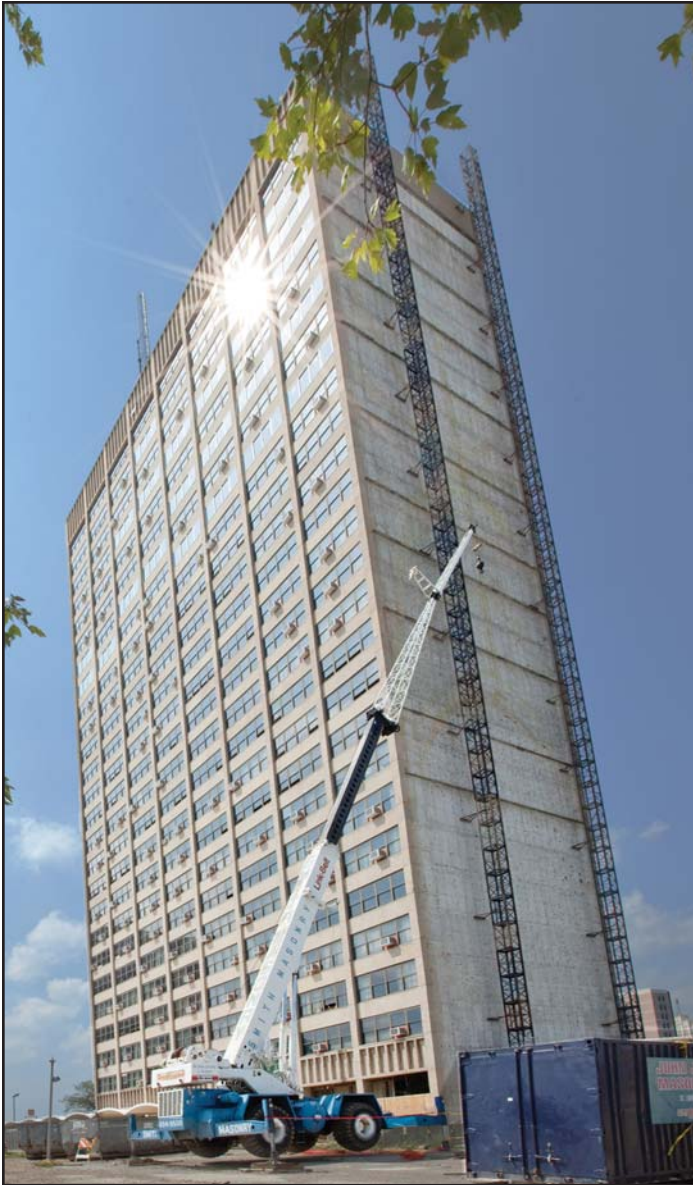
FIGURE 1. The Council Tower building in St. Louis underwent a major upgrade with the installation of a single-pipe heating and cooling system designed to save money and increase tenant comfort.
