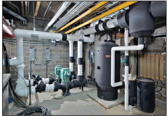
FIGURE 2. Two vertical in-line pumps, located in the basement, circulate chilled water throughout the building.
