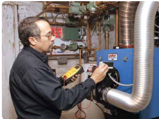
Dave Yates uses a digital multi-meter to check an oil boiler's voltage signal.
