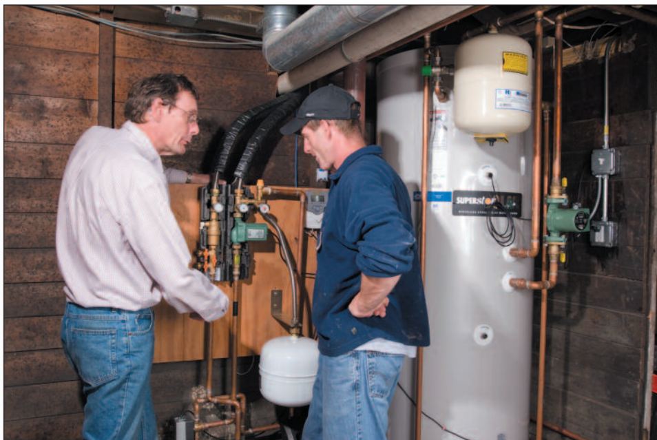
The Haverhill homeowner, left, and Ken discuss the solar thermal system's operation.
