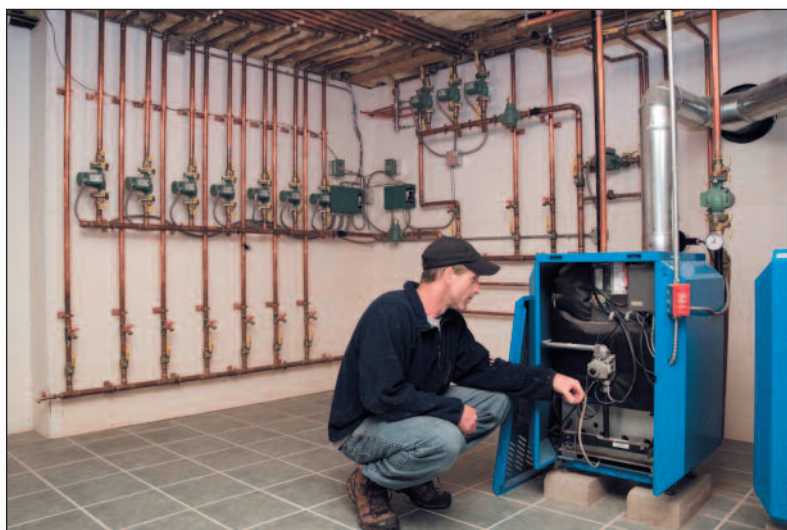
Ken Dunn, at home in his own mechanical room, checks boiler operation. The largest project Dunn's Plumbing and Heating ever tackled was a $270,000 job for a 12-bathroom, 18-zone home.
