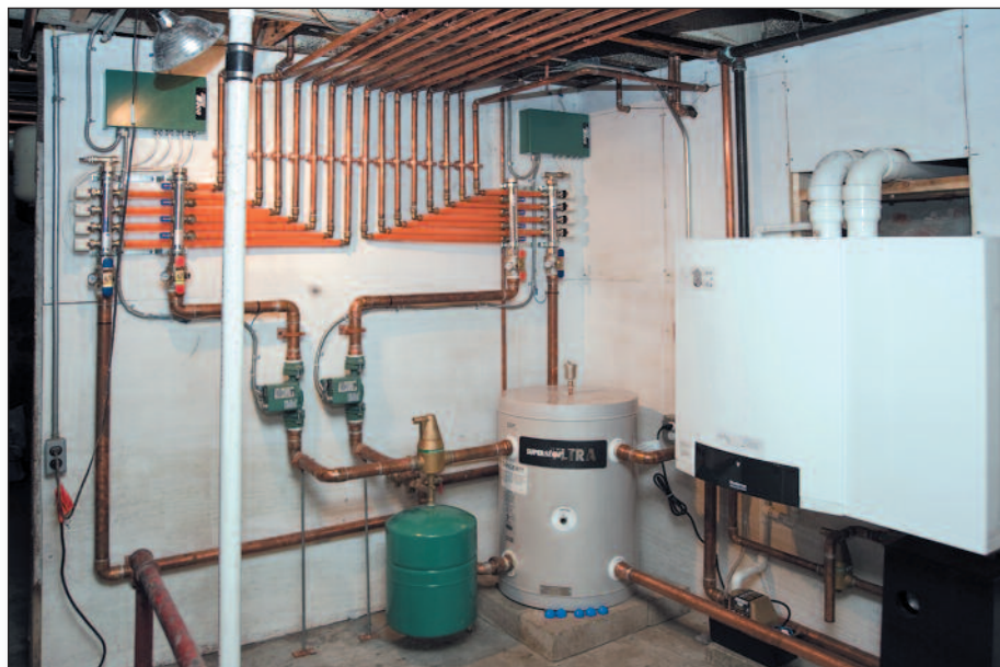
The Haverhill mechanical room is a symmetrical work of art.
