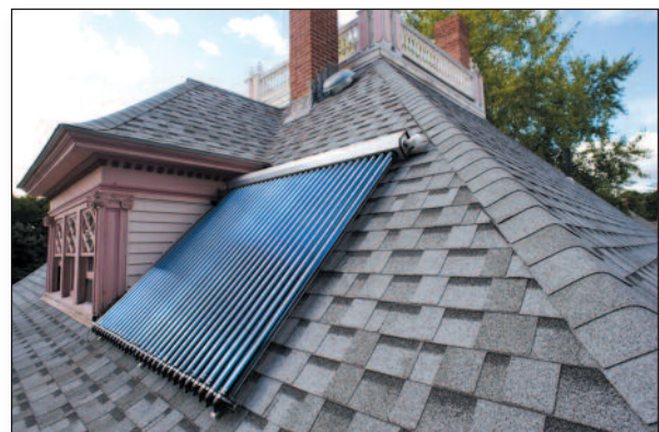
A solar thermal array installed by Ken Dunn at the Haverhill home.
