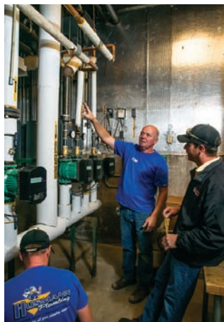
The school's maintenance room.
