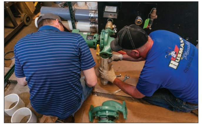
Mike Merryman (left) and Mike Husmann (right) level a Taco in-line pump on the supply side of the boiler.
