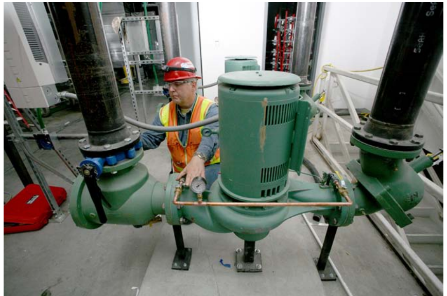
A Taco 60/13 40-hp KV vertical inline pump with Baldor Super E motor with multipurpose valves (MPVs) and suction diffusers connected to a variable-speed drive circulates water to and from a cooling tower. (Taco recommends a spool piece between the discharge nozzle of a pump and a MPV. The MPV to the right of the pump is installed incorrectly; mounting a valve directly to a pump is not recommended.)
