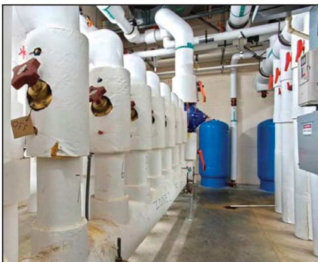
FIGURE 2. Standing column well manifolds for the geothermal system.
