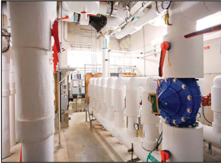
FIGURE 3. The well manifold control room.
