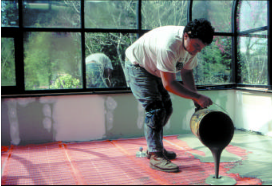
Installing the Suntouch mat was a snap. Much of the three days’ installation was spent mixing and pouring the floor’s thin layer of cement. The cement provided thermal mass and a stable floor to support the Swiss-made engineered wood surface. Contractor John Miller had never installed an electric radiant floor, but with tech help from Watts, had no problems. “Not bad for first-time installers,” Miller says.
