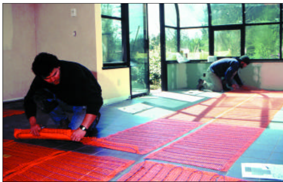
Because the garage converted into an exercise room had no boilers or other hot-water source, Miller chose electric radiant heat. A total of 560 square feet of Suntouch radiant mat provides as much as 40 Btuh/sq. ft. to the floor. The 220-volt system is controlled by seven-day a.m./p.m. programmable thermostats.
