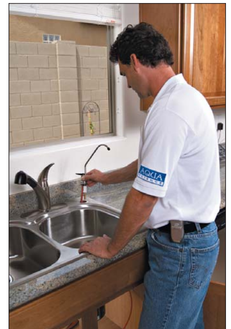
With the installation of the RO faucet nearly complete, Sajdak will test the system. This new technology could set the standard for water savings.
