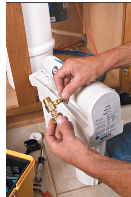
Sajdak installs the unique adapt-a-valve for the cold water connection. All of the concentrate water from the RO system is routed to the hot water supply via a fitting on the angle stop valve.
