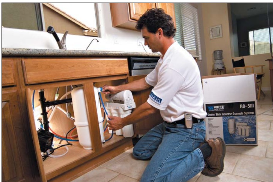
Sajdak connects the water storage tank. The ZeroWaste System returns the concentrate water from the RO system back to the home's plumbing, resulting in 100% efficiency.
