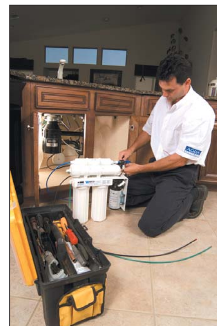
Derek Sajdak prepares a ZeroWaste module for installation. The system reduces the amount of water to produce one gallon of product water.
