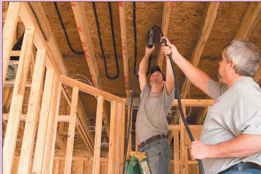
Technicians with Freeland Contracting Co. staple up a radiant floor using Watts Radiant Onix tube. They chose Onix because its rope-like flexibility allows easy installation between floor beams where installing PEX would be a "wrestling match."
