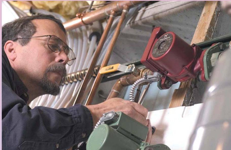
Use one pump and select the speed to match the flow and head you want. In large radiant heat installations multi-speed circs provide the ability to balance water flow to each manifold no matter how many loops are on it.
