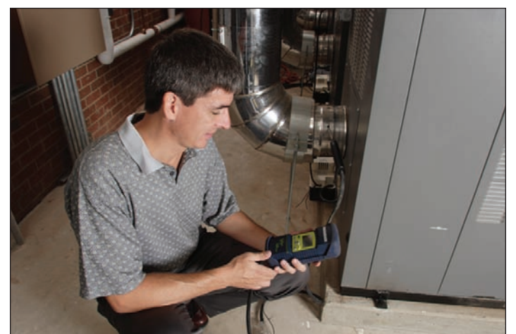
Tod Hebert, Northeast regional sales manager for Laars uses a combustion analyzer to assure optimal combustion (the device measures CO 2 , CO and flue temperature, among other functions).
