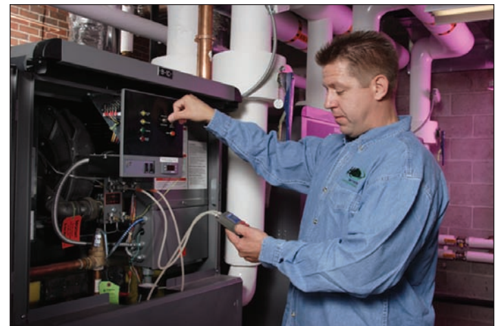
Dave Warzecha, onsite project manager for P&D Mechanical, uses a manometer to check boiler gas pressure differential to verify that the combustion gas-to-air ratio is correct.
