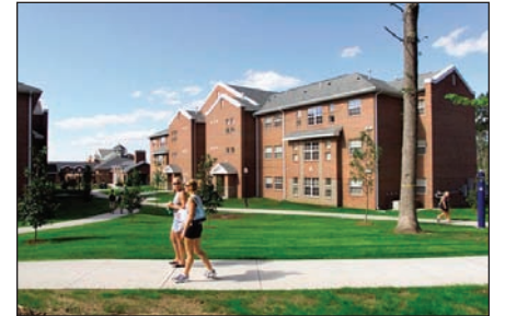
P&D Mechanical, Inc., Colchester, Conn. replaced the heating/hot water systems in Hilltop Apartments' 12 student housing units at the University of Connecticut, all during the summer when students weren't in residence.
