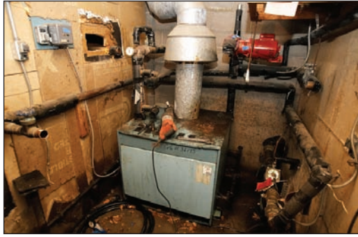
The complex's 6'x10' boiler space presented a challenge to Advanced technicians, who turned this shambles into a neat, organized mechanical room.
