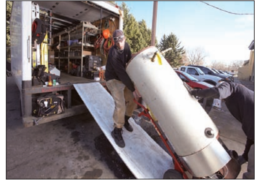
Advanced techs load up an old, leaking water heater, to be replaced by a 120-gallon Bradford White indirect water heater coil.
