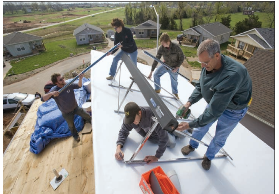
Bob "hot rod" Rohr and students install an Apricus 30-tube vacuum solar array on the roof of Drury University's Sustainable Habitat House project in Habitat for Humanity's Legacy Trails subdivision north of Springfield, Mo. During winter months, the solar array will heat a propylene glycol solution to about 110°F.
