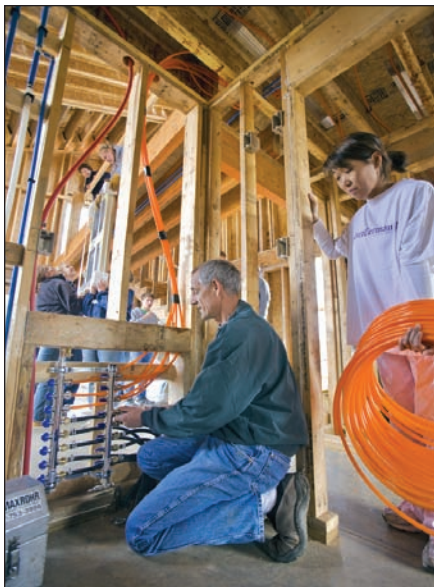
Hot Rod instructs a student in the intricacies of installing radiant manifolds for the home's two zones.
