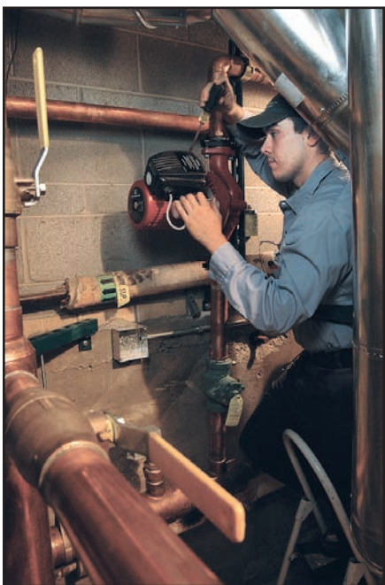
ACA Denver Boiler installed Grundfos 3-speed pumps at a LDS church project.
