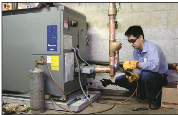
A check valve is installed on the boiler loop piping at the Sherman Street Apartments.
