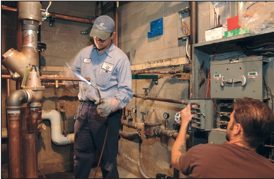
While doing a boiler replacement for a local LDS church, an HVAC apprentice prepares piping for installation of two Pennant hot water heating boilers. Meanwhile, an electrician prepares the wiring for the boilers.
