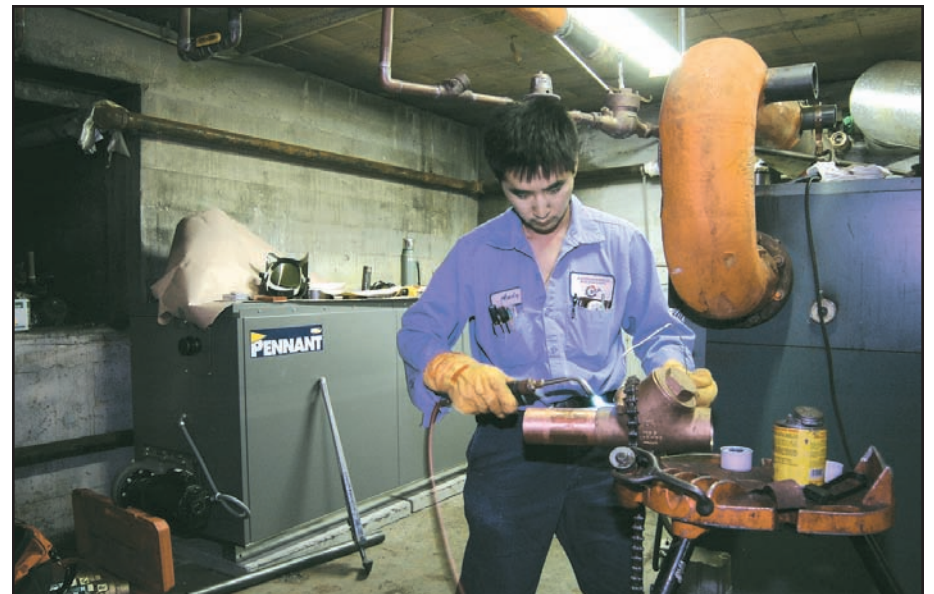
At the Sherman Street Apartment complex, an apprentice solders a 2 1 / 2 " check valve for installation of one Pennant hot water heating boiler.
