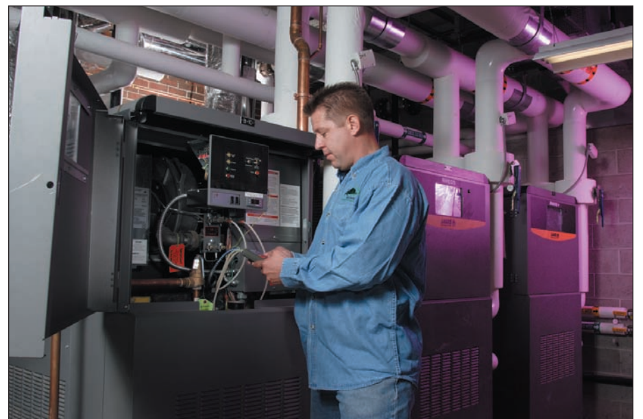
Dave Warzecha, P & D Mechanical project manager, performs a system diagnostics for a multiple Laars Rheos high-efficiency boiler/volume water heater installation at the University of Connecticut.
