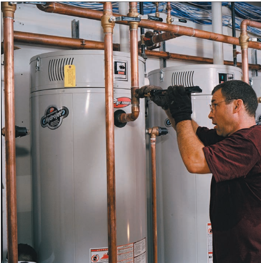
A Family Plumbing technician completes a Bradford White eF water heater installation at a new hotel in New Jersey.
