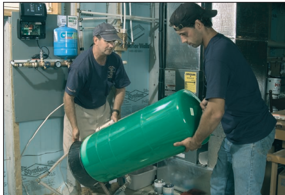
A free-standing, 20-gallon storage tank was removed in favor of a much smaller, two-gallon tank that was hung on the wall (blue tank in background), saving space in the basement mechanical room and saving costs on the front end.
