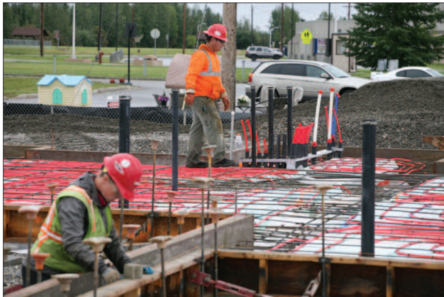
Eielson Air Force Base undertook the construction of 349 new, multiple-family housing units (or multiplexes), and 99 existing units received mechanical system upgrades, all completed by Slayden Plumbing and Heating.
