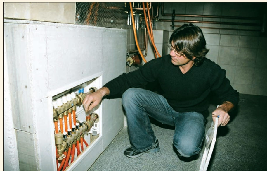
The home's 12-zone, multi-temperature hydronic system employs multi-speed circulation and Grundfos SuperBrute pumps, while Caleffi zone valves and an insulated Hydro Separator enable the primary and secondary loops to operate hydronically independent of each other.
