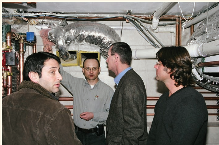
From left, Mike Bleier, Piotr Zelasko, John Siegenthaler and Zbyszek "Ziggy" Jonak examine part of the comprehensive radiant system Ziggy retrofitted in his 70-year-old, 5,400-sq.-ft. home in Highland Park, Ill., north of Chicago.
