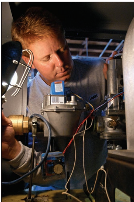
A technician examines the inner workings of a Laars boiler.
