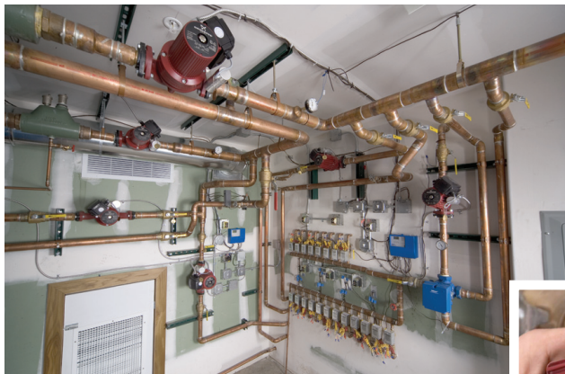
Pictured above is Avon, Co.-based Concept Mechanical's mechanical room with several multi-speed VersaFlo circulators installed.
