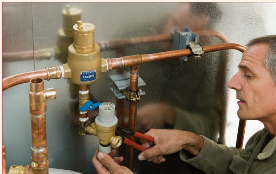
Bob “hot rod” Rohr installs a caleffi fill valve below the air eliminator.
