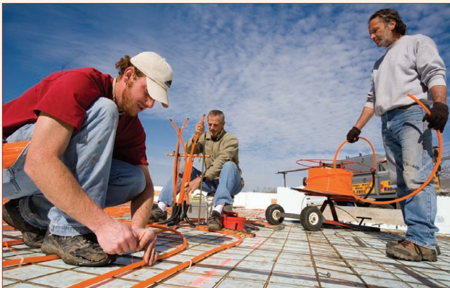
Contractors lay down about 2,700 lineal feet of Watts Radiant’s RadiantPEX in just two heating zones embedded in heavy concrete.
