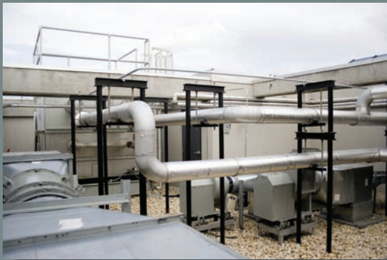
Water-source heat pumps easily reject unwanted heat through cooling towers.
