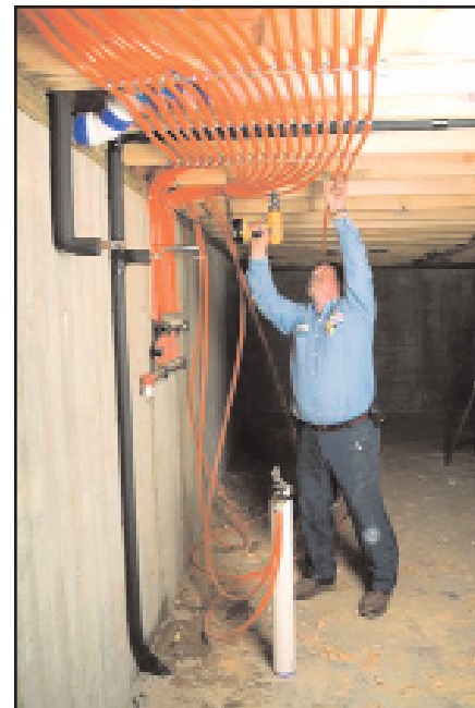
Oren Atchley Co.'s David Kuykendall installs RadiantPEX to the manifold. About 12,000 lineal feet of the tubing was used for the project.
