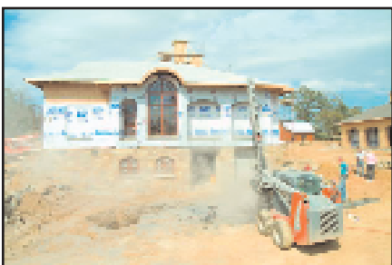
Contractors drill holes for the geothermal heat pump system during construction of this magnificent 8,000-square foot home.
