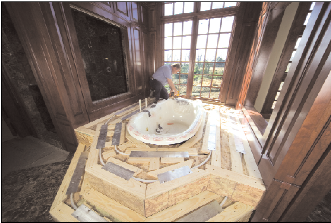
Combining radiant heat with alternative energy and/or ultra-high-efficiency heat sources puts 'the best of both worlds' together. This 8,000-square-foot luxury home took 38 months to complete. Contractors linked six geothermal heat pumps with an extensive 10-zone radiant heat system that has all the bells and whistles. Here, Oren Atchley Co.'s David Kuykendall installs RadiantPEX and plates in what may be the ultimate, radiantly heated tub-surround. See the full story on page 31.
