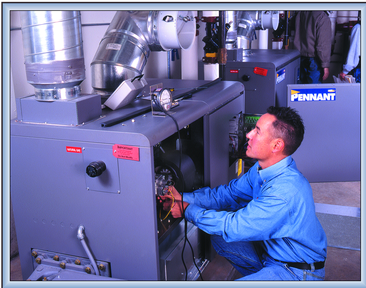
Recent boiler replacement project at Shoreline Community College, near Seattle, Wash., saw manufacturers' representative Columbia Hydronics of Vancouver, Wash., work closely with mechanical contractor McKinstry Co. in engineering and supplying the job with two fan-assisted, sealed combustion boilers from Laars Heating Systems. Here Columbia technician Mike Petterson verifies gas line pressure during startup.
