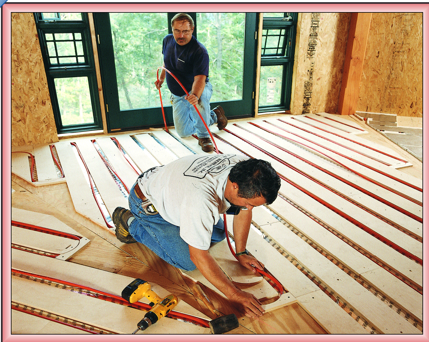
Since comfort is quintessential to any heating system, radiant floor heat simply can't be beat. But proper installation is critical, so every link in the supply chain must be competent. Here Dave Yates (foreground) and Scott Barnett of heating contractor of F.W. Behler Inc., York, Pa., lay Watts Radiant's modular SubRay hydronic flooring panels sourced from full-service plumbing/hvac wholesaler York (Pa.) Corrugating Co.
