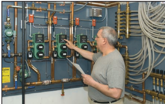
Homeowner/system installer Steve Taber sets parameters for one of four Taco Radiant Mixing Blocks. Each device offers complete injection mixing, combining a variable speed injection mixing control, injection circulator, system circulator and air elimination in a single unit.
