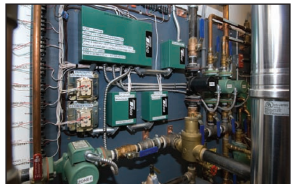
Car restorer Taber put his talents to use designing and installing his professional-looking radiant system.
