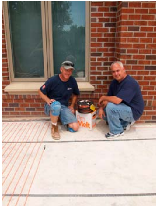
Mark Walz of Walz & Floors and Joe Abramo of The Floorplan, the Omaha-based contractor who installed the ProMelt system.
