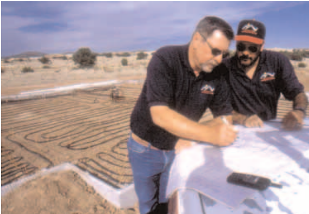
Sun Mountain Plumbing President Michael Richardson (left) and field foreman xxxxxxxxxxxxxxxx double check the tubing runs on a new construction project just outside of Santa Fe.
