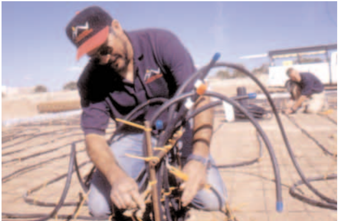
Radiant tubing is laid out in 200-ft. runs, creating a self-balancing system. The ends are manifolded as shown here so that the boiler plant can be quickly installed after the home is framed.
