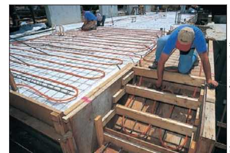
Stairs are another excellent application for radiant snowmelting, providing an extra measure of safety.
