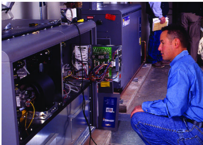
After the Pennant boiler is fired, Mike checks temperatures at the system's internal control board.
