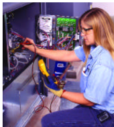
McKinstry technician checks voltage to a gas valve in the Pennant boiler.
