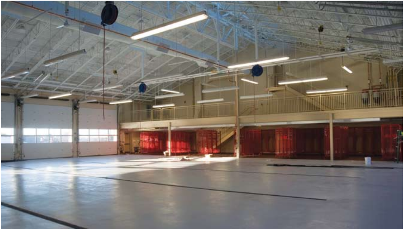
At floor level, the large bay shows no sign of heat within the slab. An infrared photo at this angle, however, would reveal the "secret" of radiant warmth below. The network of tubing also extends into the large concrete pads outside, assuring safe and rapid exit any time of year.
