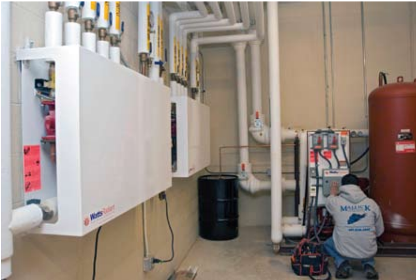
A Mallick technician performs prefire diagnostics on the system.
