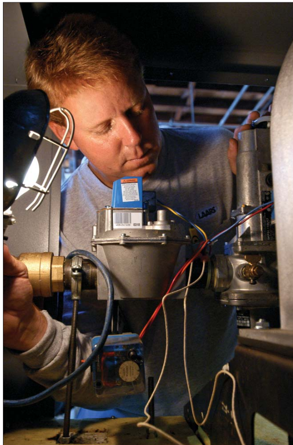
Mike Elmore, LAARS territory service manager, inspects a Rheos boiler/water heater at the U.S. Water Polo National Training Center in Los Alamitos, CA.
