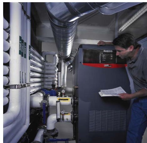
Kevin Michel, president of Gardena, CA-based Xcel Mechanical, examines the installation of a Rheos boiler at Mammoth Mountain ski resort.
