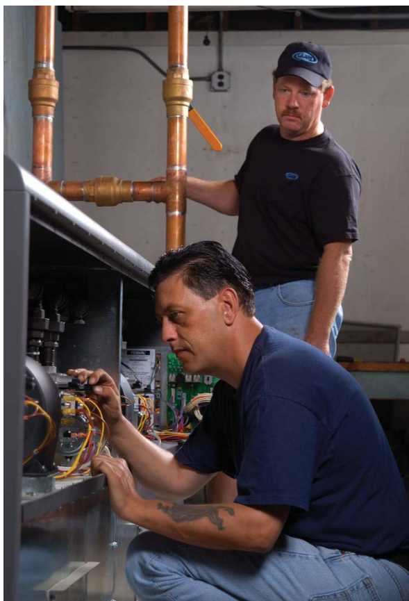
A Pennant boiler gets a pre-fire inspection at the Los Alamitos Olympic pool facility.
