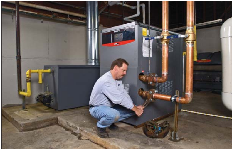
High-efficiency Pennant (left) and Rheos (right) boilers are prepared for start-up prior to heating the Olympic pool's 649,000 gallons of water, now at an annual savings of $5,000.
