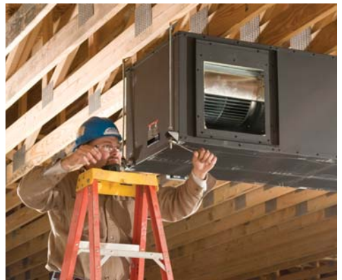
This light commercial application places a geothermal air handler just above ceiling tiles in a new restaurant.
