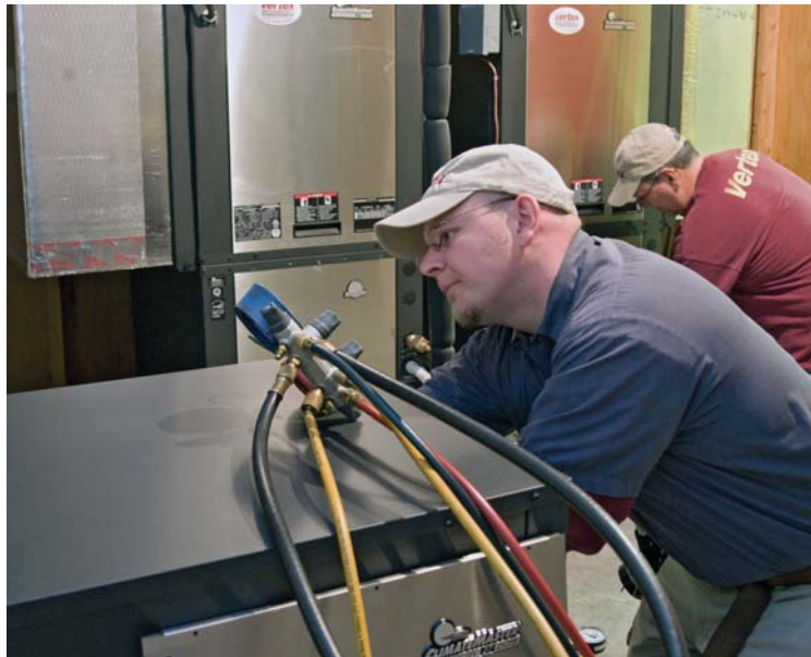
This new geothermal system meets a large home's HVAC needs year 'round while supplying most of the domestic water heat as well.
