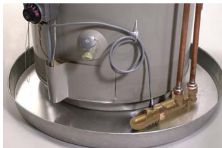
An installed WAGS shut-off valve from Taco is added assurance against water heater leakage.
