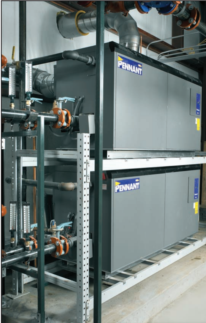
FIGURE 2. Two 1.5 million Btu, fan-assisted boilers are at the heart of the radiant heating system. The units operate at 85% efficiency with four-stage control to meet demand.
