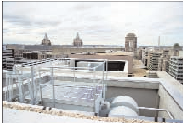
From a rooftop perch, the Washington Monument is seen beyond the Alta's cooling towers.
