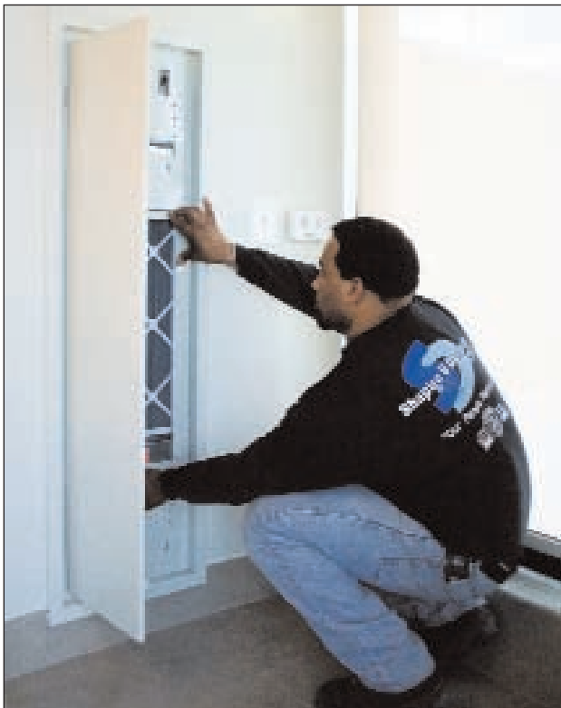
A technician completes the installation of a TRM vertical stack unit in the Alta at Thomas Circle, Washington, D.C.
