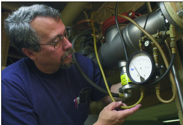
Care should be taken to insure that adequate floor drain capacity is specified to allow the discharge of water from the relief valve of the RPZ
