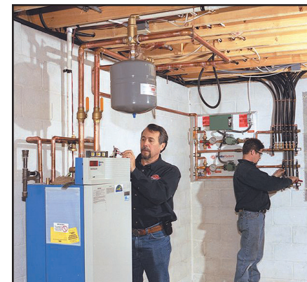
An LP-burning Laars Endurance water heater/boiler provides heat and domestic hot water — far more than the old electric water heater did.
