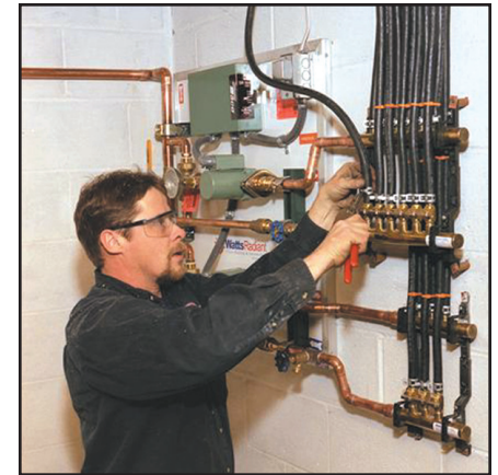
A Watts HydroControl panel regulates two zones and eight loops; a three-way mixing valve tempers water as needed.
