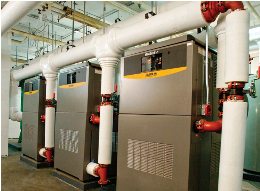
(Top, left to right) Steve Schneider, Frank Zieris and Ike Beyer inside one of Spring Creek Gardens' six boiler rooms. (Above) Integrated HVAC installed a total of 18 Laars Rheos+ boilers ranging in size from 1.2 million to 2.4 million Btu.
