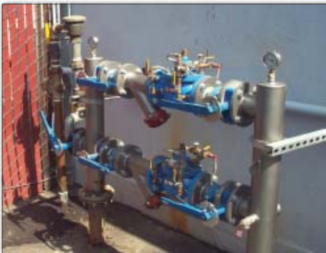
A dual 3" regulator station retrofit of an old station. Previously, the old station created a huge pressure drop in the line. But with this retrofit, the problem has been fixed.
