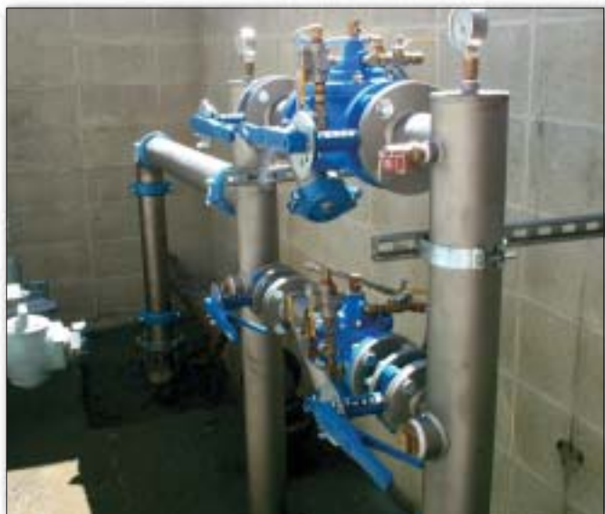
A retrofit of an old regulator station within the Los Angeles Unified School District. Pictured are dual, parallel regulator stations with 4" galvanized lines.
