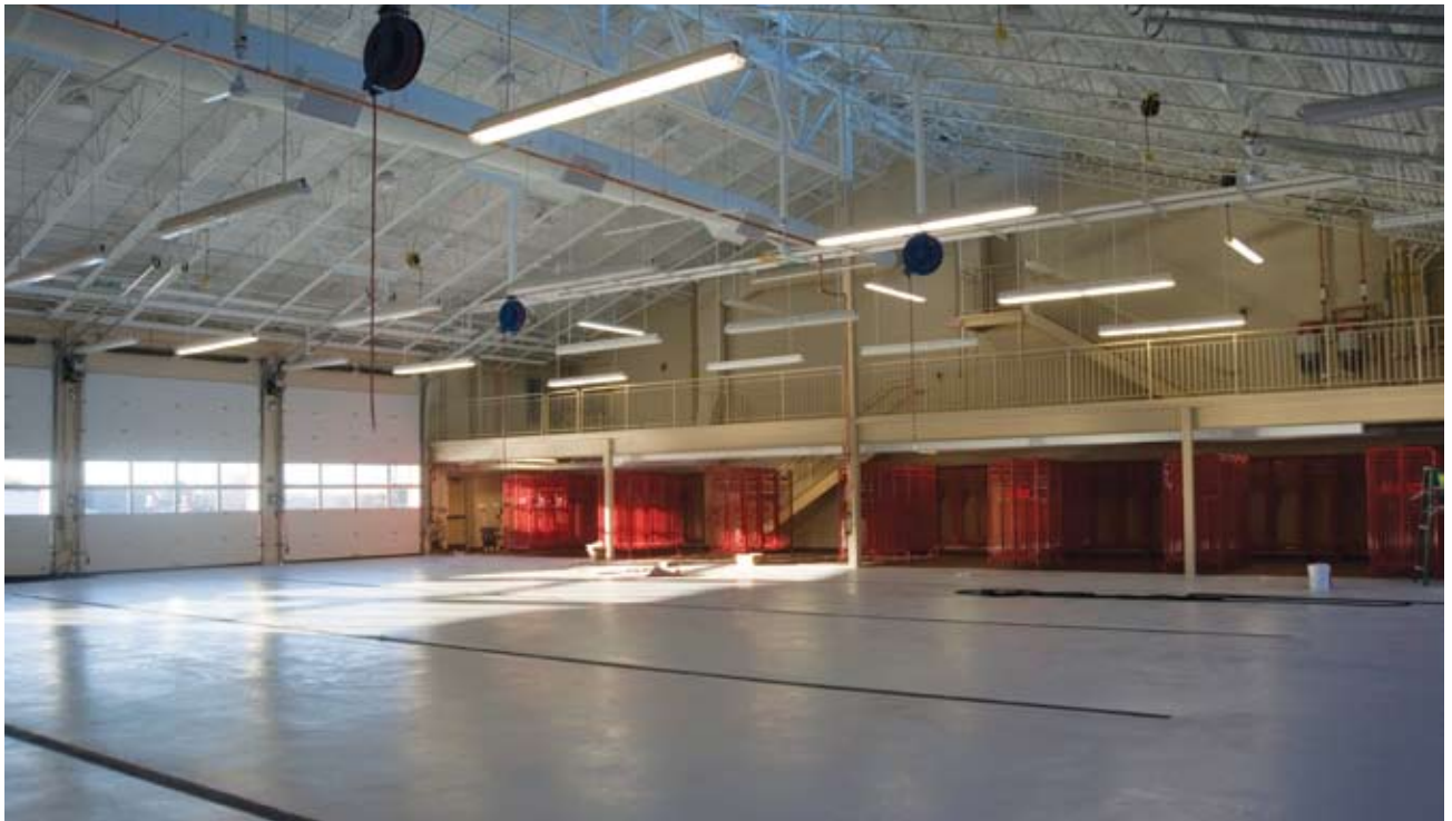
At floor level, the large bay shows no sign of heat within the slab. An infrared photo at this angle, however, would reveal the "secret" of radiant warmth below. The network of tubing also extends into the large concrete pads outside, assuring safe and rapid exit any time of year.
