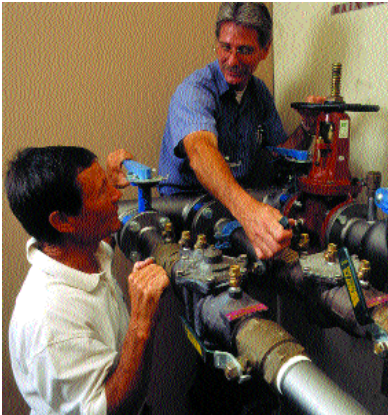
Backflow prevention expert Bernie Clarke (left), and David Sullins, chief engineer for Desert Island, make a few adjustments at the valve station located in a condo garage.
